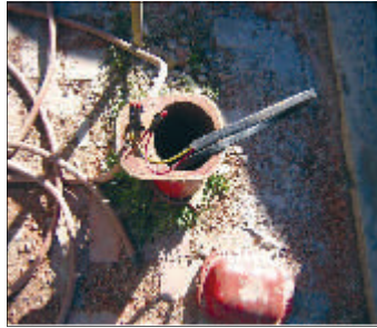
Wellhead with cover removed
