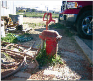
Wellhead with cover in place
